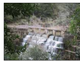
Fig. 2. Searsville Dam is an old concrete structure whose construction by the Spring Valley Water Company was first completed in 1892. Downstream releases are exclusively via the broad-crested overflow spillway weir.
