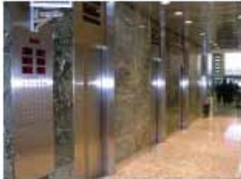
Turn off 1 of 4 elevators
